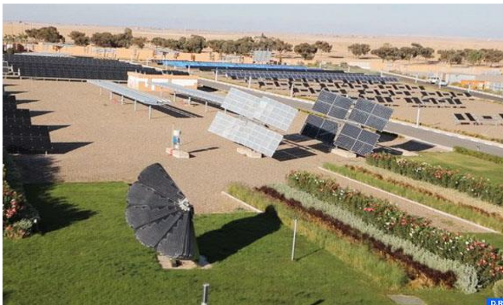
Figure 6: Green Energy park of Benguerir using the solar system [17]
